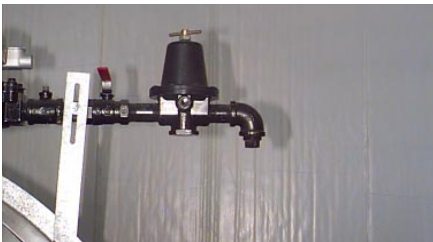
NG line field connection.
